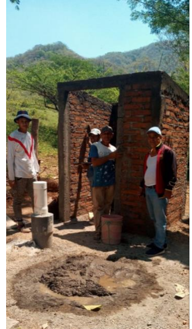
Member of the community are working in the well facilities improvement in Las Pilas Centro, El Sauce
